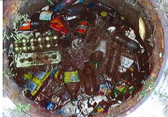
Fully Clogged basket
